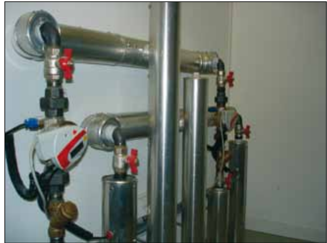
Figure 1. Heat meters with M-Bus interface and M-Bus-KNX-Gateway
